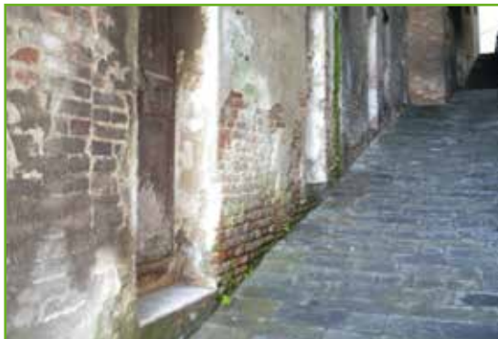
Destruction of render and mortar joints
