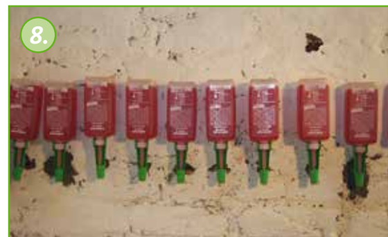
8. The pressureless injection of KÖSTER Crisin® 76 into the masonry starts immediately after the installation of the cartridges.
