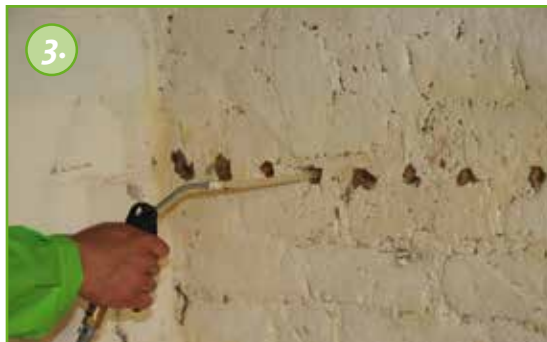
3. The boreholes are cleaned from dust by blowing the dust out of the borehole with pressurised air.
