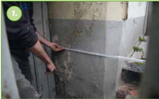
1. The masonry is from 1750, the existing plaster is damaged. The salt and moisture contents are high.
